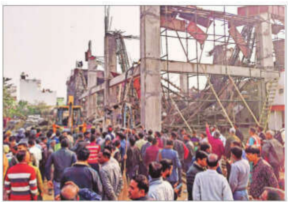
Rescue operation underway after an under-construction building collapsed at the Kannauj railway station, trapping around two dozen workers under the rubble on Saturday afternoon
