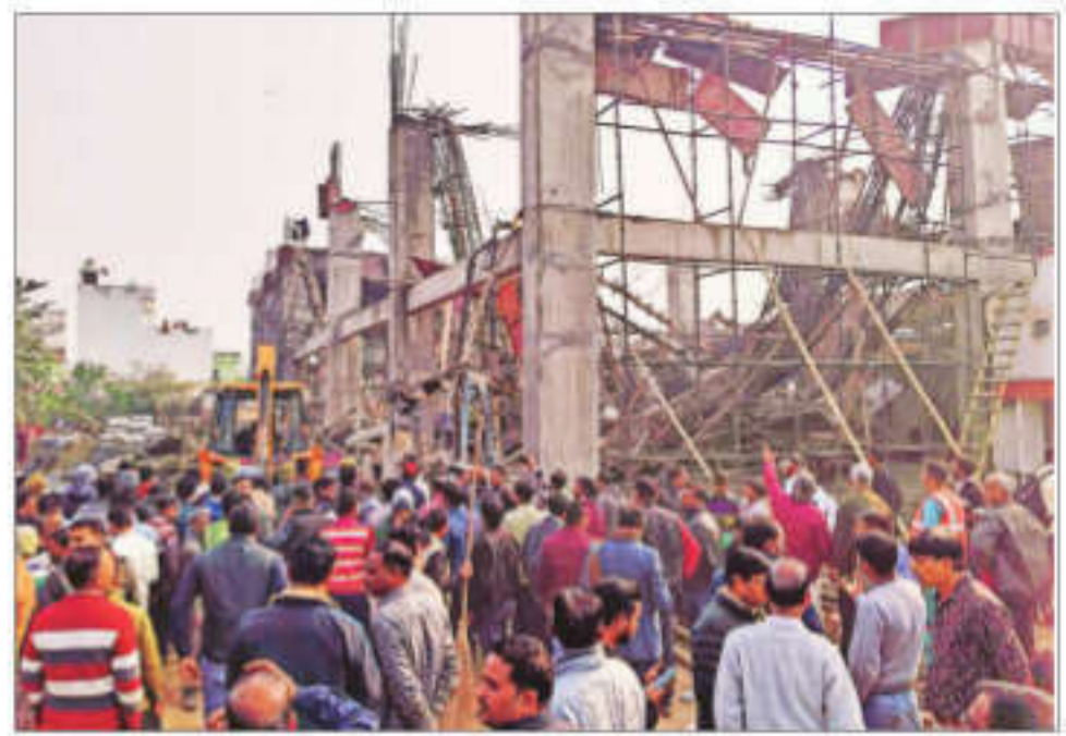
Rescue operation underway after an under-construction building collapsed at the Kannauj railway station, trapping around two dozen workers under the rubble on Saturday afternoon
